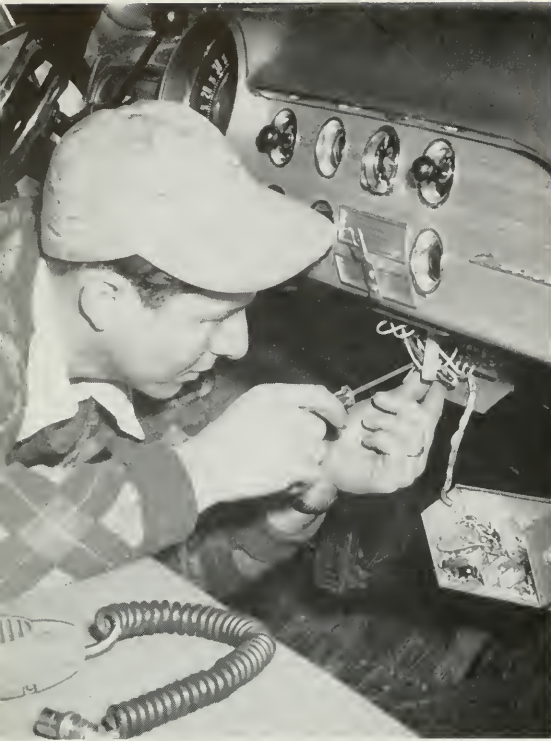
Installation of mobile two-way radio systems is an important RCA Service Company job.
